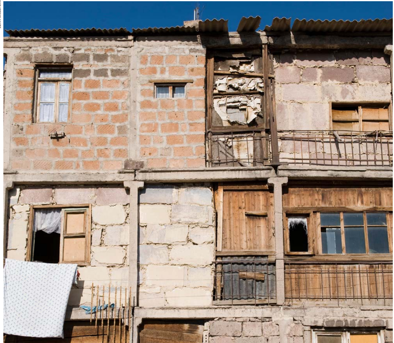
A crumbling Soviet-era apartment building.
